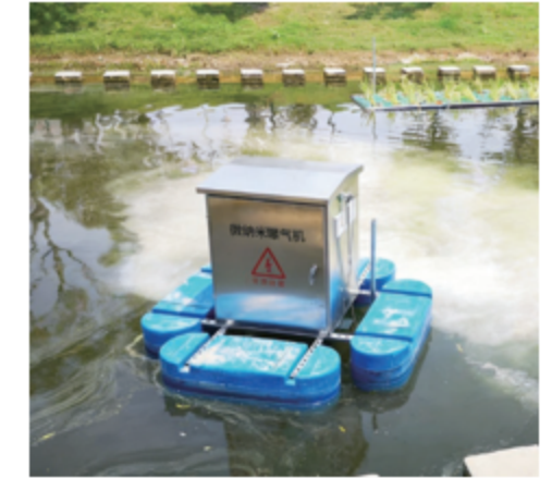
Micro-nano Aerator Installation Site
