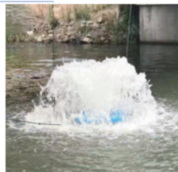
Spring Aerator Installation Site
